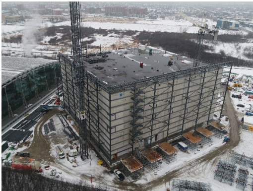
LAC's future Preservation Storage Facility under construction in 2020. Photo: Plenary Properties Gatineau
